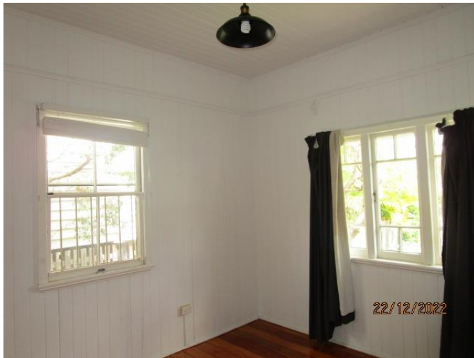
35. The bedrooms were well presented. The timber joinery windows require servicing.
