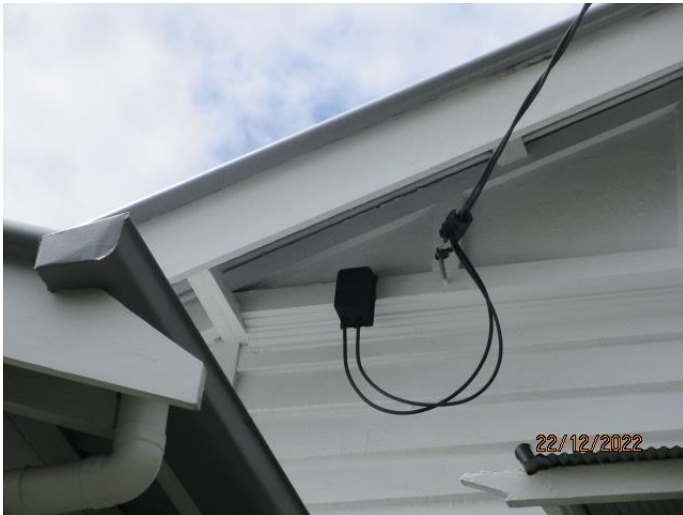
6. The overhead power connection was secure.
