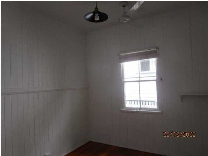
39. The second bedroom is in good condition. The windows require servicing. The cladding has no evidence of any major damage.
