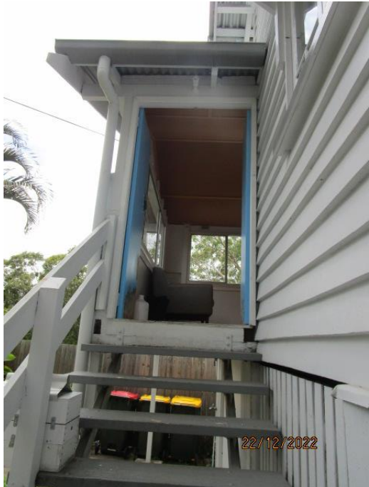
27. The entry door functions and locks. The entry doors require rejuvenation as they have scratch marks.
