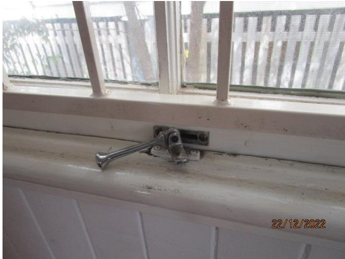
36. The timber joinery windows do function but require servicing and paint maintenance.
