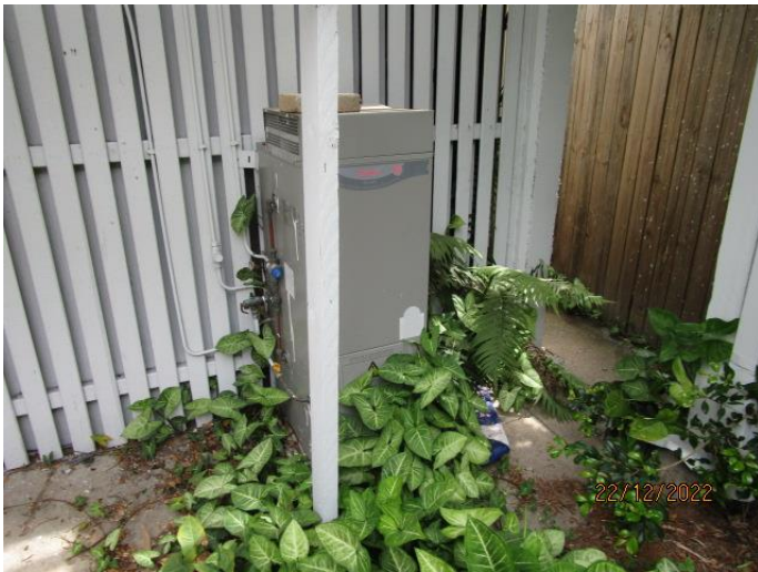
20. The gas hot water unit functions. I recommend all appliances are serviced. The vine climbing around the hot water unit requires removal.
