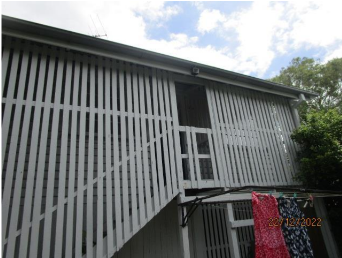
19. The privacy screens require maintenance. The balustrade in the centre requires repairs as it is considered a fall hazard in current form.
