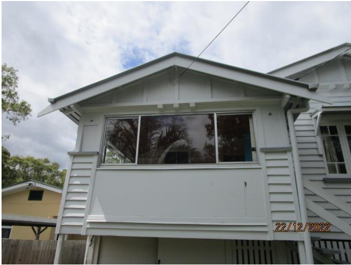
5. The exterior of the home does have some imperfections. There is no major damage. This front panel underneath the window does have damage on the inside and requires repairs. This is an enclosed balcony. The overhead telecommunications bracket was secure.
