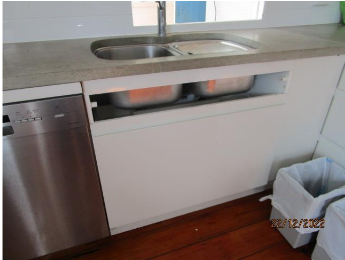
45. The panel at the front of the sink requires reinstating.
