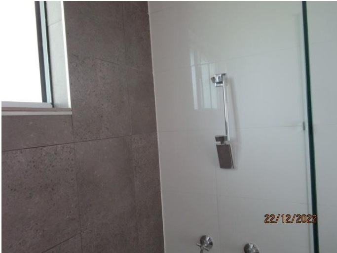
57. The shower plumbing functions.
