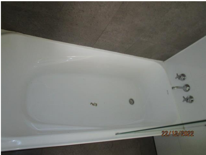
56. The bath plumbing functions. Underneath the bath has evidence of a water leak. This was not leaking at the time of the inspection.
