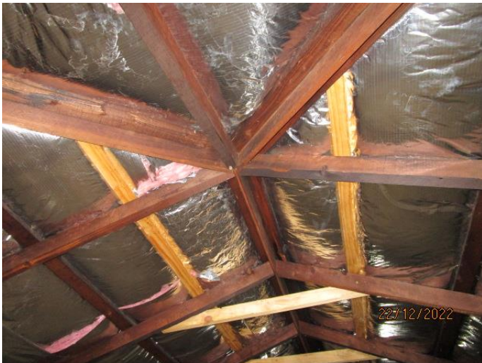
62. The roof structure was in very good condition. There is a moisture barrier and installation underneath the roofing iron.
