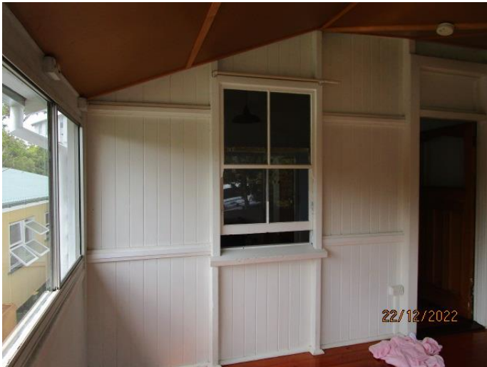
30. The front of the house is quite well presented. All timber joinery windows and doors require servicing.
