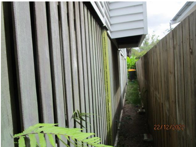
21. The fences were in quite good condition. The lower-level exterior tickets were in quite good condition. The base does have some damage.
