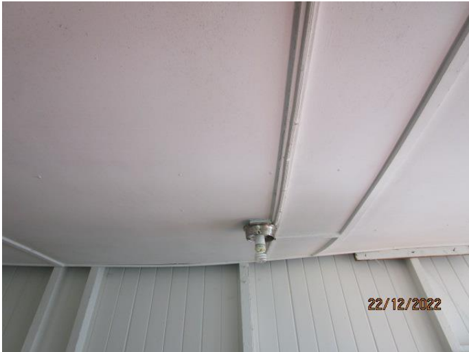
61. The ceiling in the enclosed balcony central area has released itself. This requires pushing back up with additional nails and screws.
