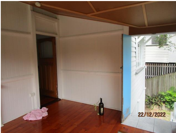
29. The doors require rejuvenating.
