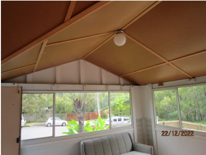
28. This is an enclosed balcony. The front wall has damage and require some repairs. Craft wood ceilings have been installed in the entry.
