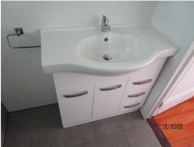
55. The vanity sink and tap had no leaks. The cabinet was in good condition.
