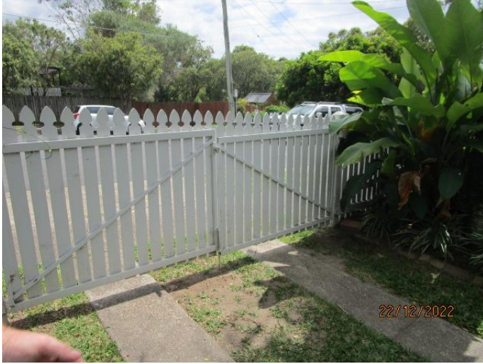
4. The gates require slight adjustment. The driveway tracks were in quite good condition.
