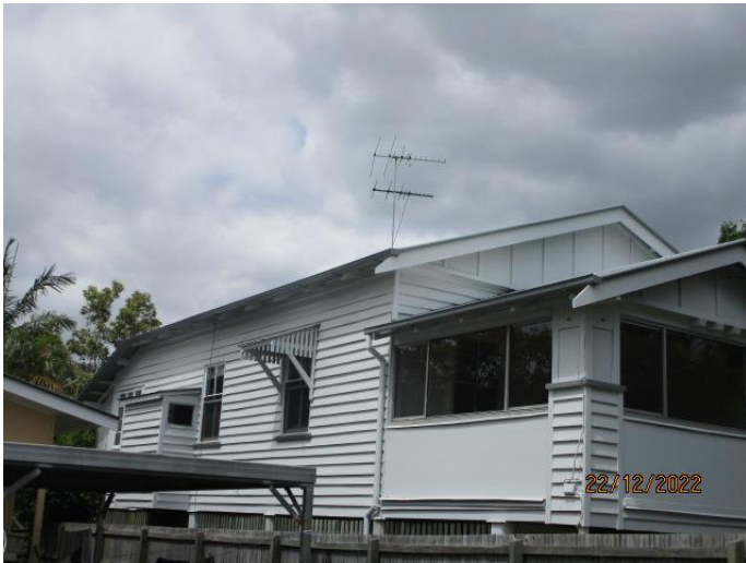
65. The exterior of the home in general was well presented. There are some imperfections but there is no evidence of any major damage.
